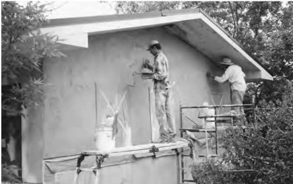
8-11: Worker troweling lime plaster on wall. Be sure to wear goggles or glasses, gloves, and cover up the rest of your body.
