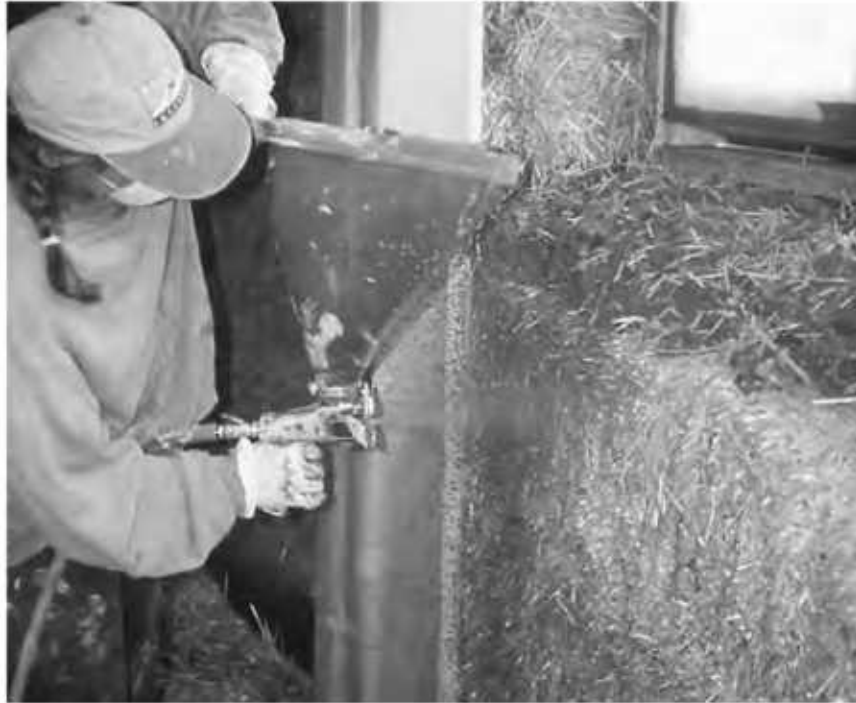
6-4: Clay-slip can be sprayed onto straw bale walls using a drywall texture gun which ensures that it penetrates the surface of the bales.
