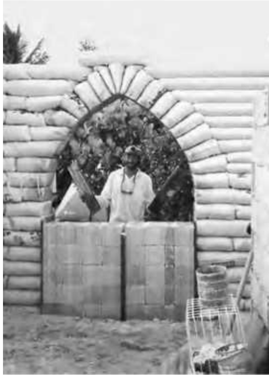
1-14: Earthbags placed over forms create wonderful arches for windows, as shown here.
